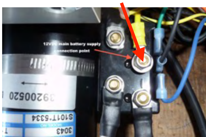
MAIN +12VDC POWER from house battery
